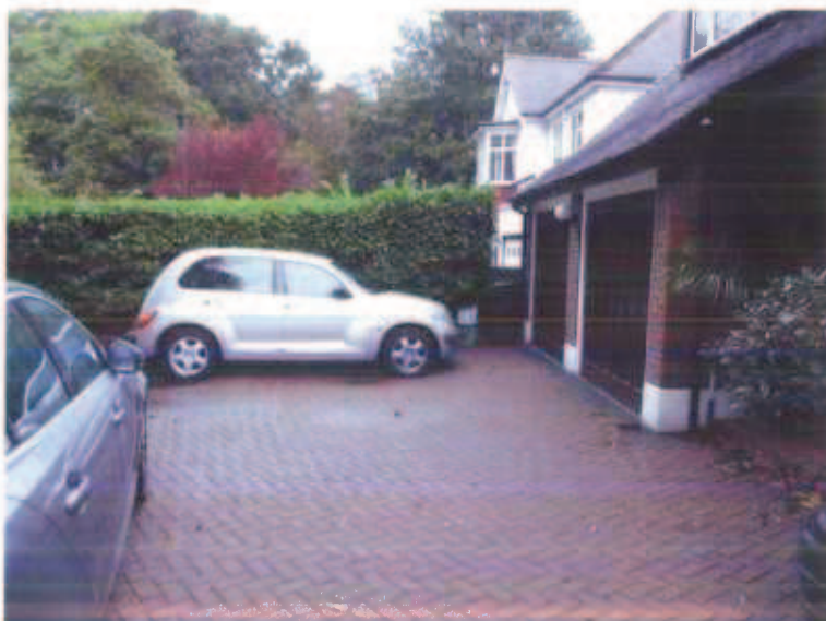
Photograph 6. View looking to the north across the front of No.12 showing the block paved drive.
